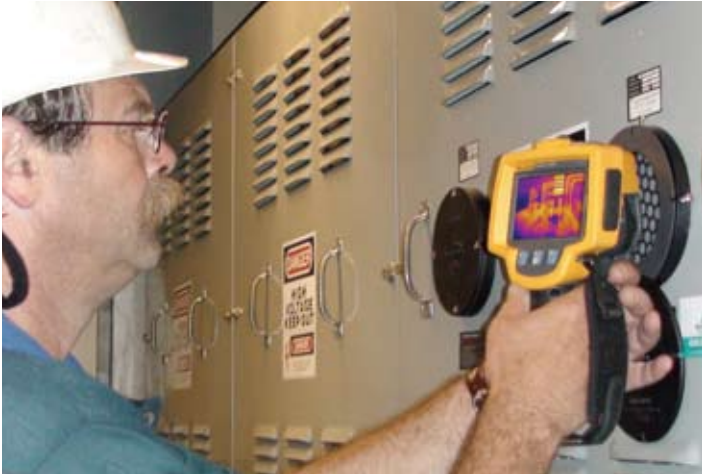
Example of a thermographer using an IR window and wearing standard level of PPE required while operating energized electrical equipment in an enclosed and guarded condition.
